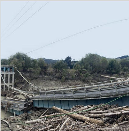
Hikuwai bridge on SH35, which runs along the East Cape north of Tolaga Bay, after Cyclone Gabrielle in February 2023
