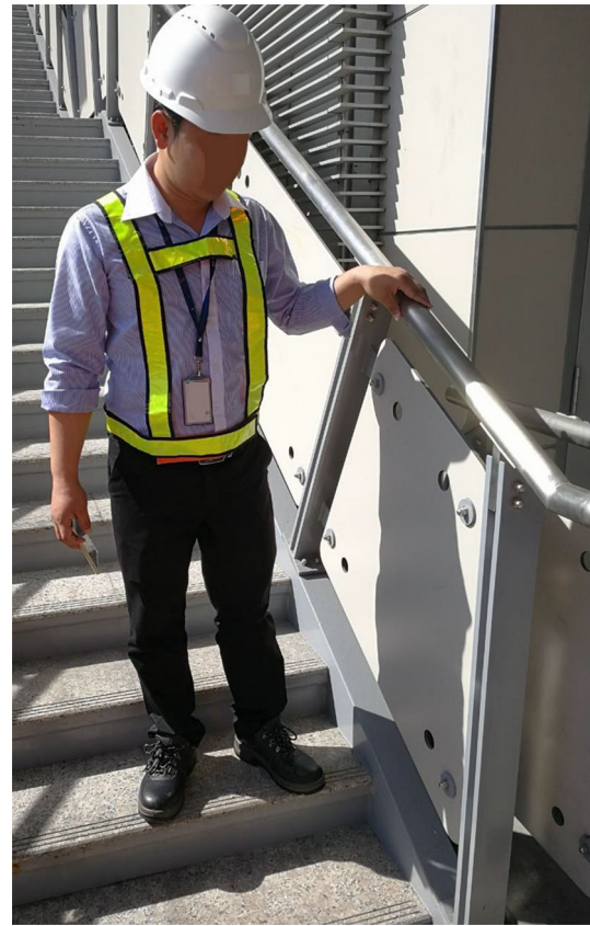
Fig. 4 Design and construction of handrails at a height of 1220 mm with 50-mm tubing due to misinterpretation of design standards, posing a hazard and increasing risks to children and the elderly
