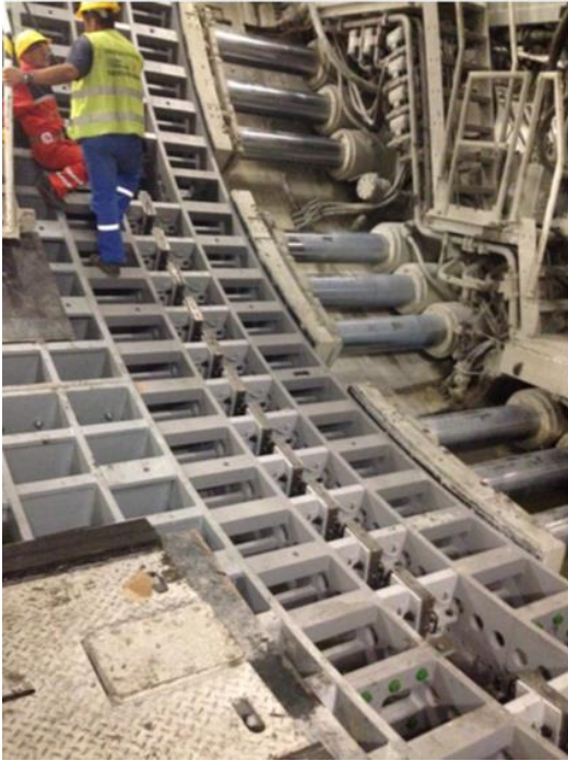
Figure 5 - Special seismic joint installed in the Eurasia Tunnel
