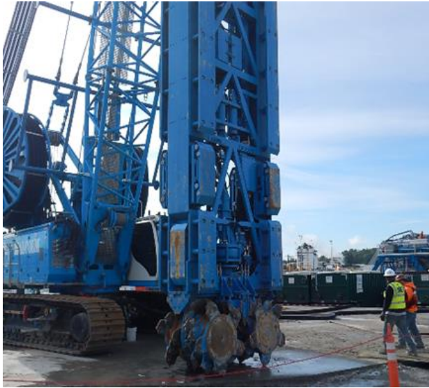
Figure 2 - Excavation of interlocking slurry wall panels in weak ground to create tunnel boring machine (TBM) launch shaft.
