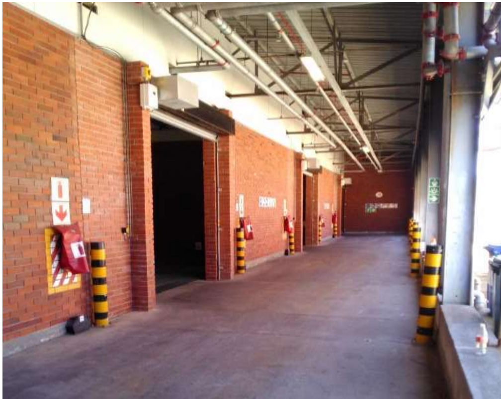
Figure B : Internal view of the roller door from the corridor within the Flammable Drum Store.
