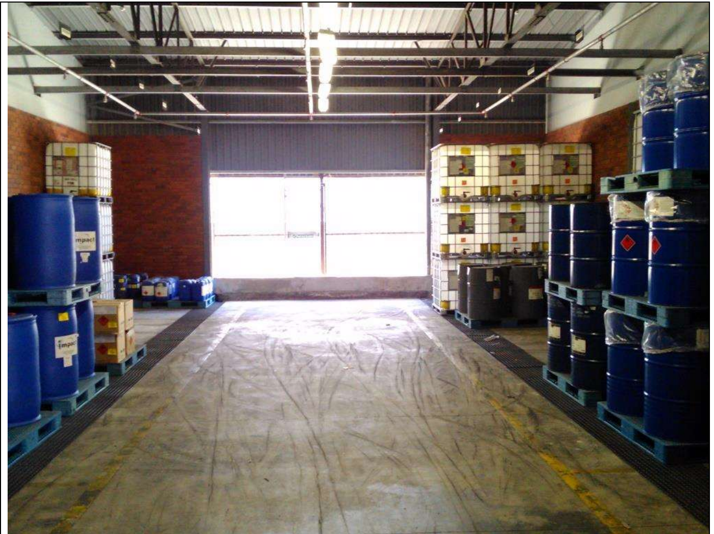
Figure A : Internal view of the Flammable Drum store which has been upgraded.
