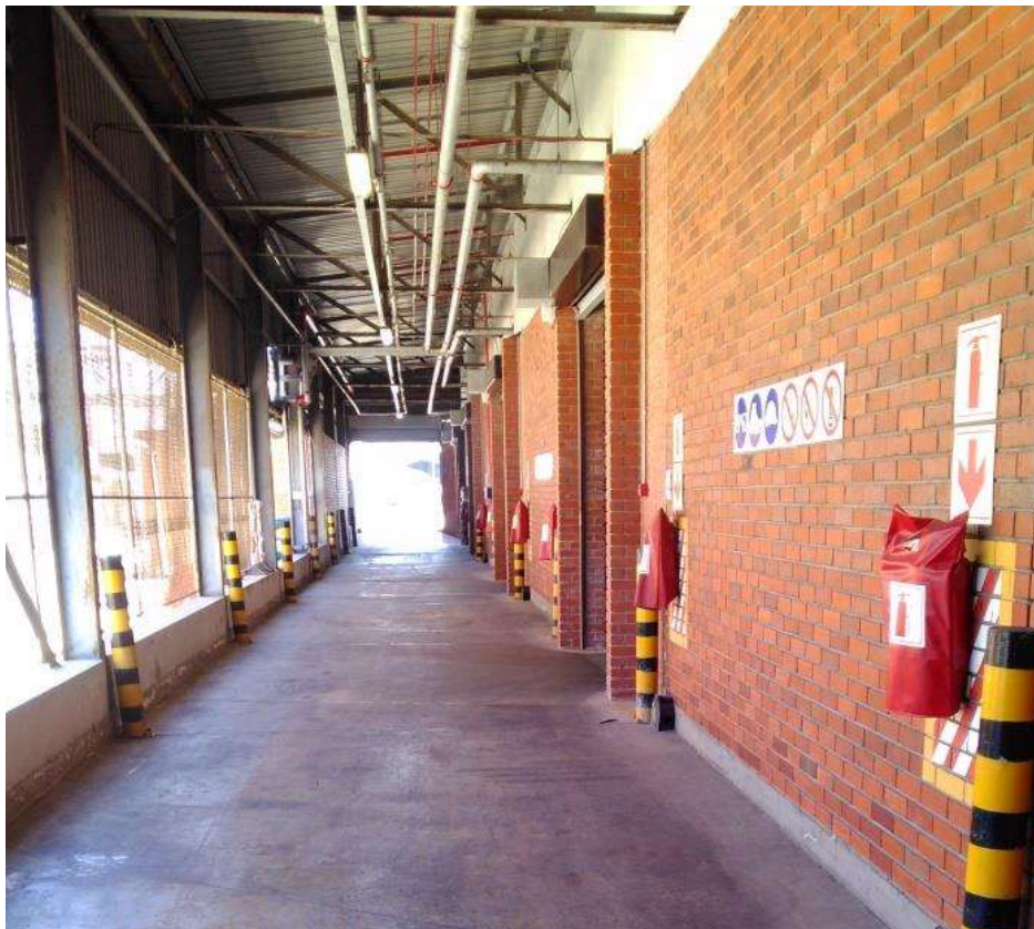
Figure D : Internal view of the corridor and bunding surrounding the flammable storage facility.
