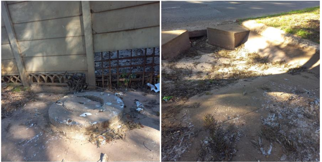
Figure 5-4 - Blocked manhole discharged into the stormwater channel
