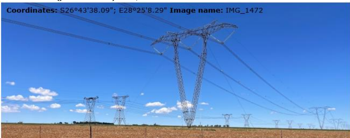
Figure 7-110 - Existing power lines within the study area
