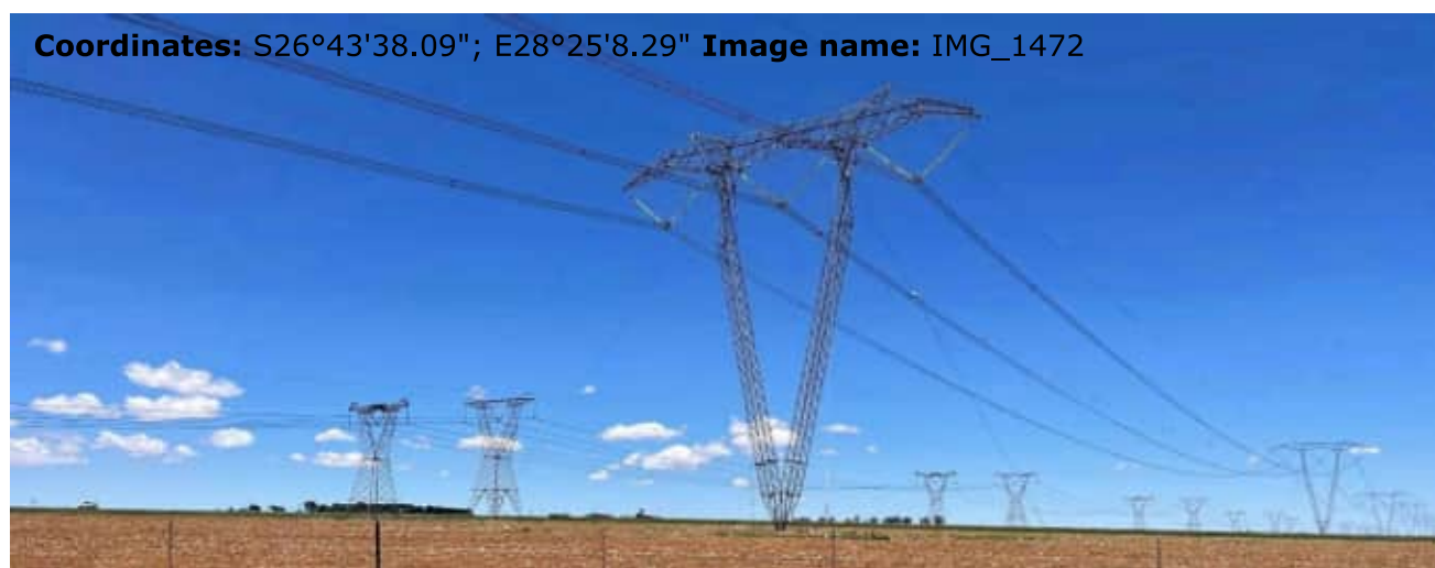
Figure 8: Existing power lines within the study area
