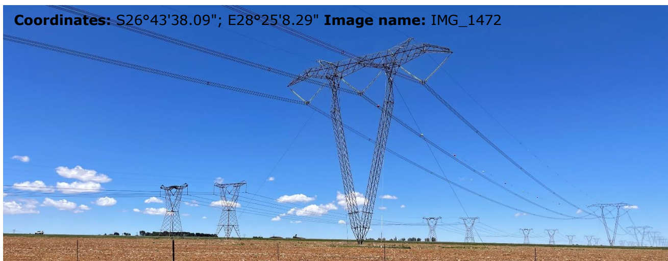
Figure 8: Existing power lines within the study area
