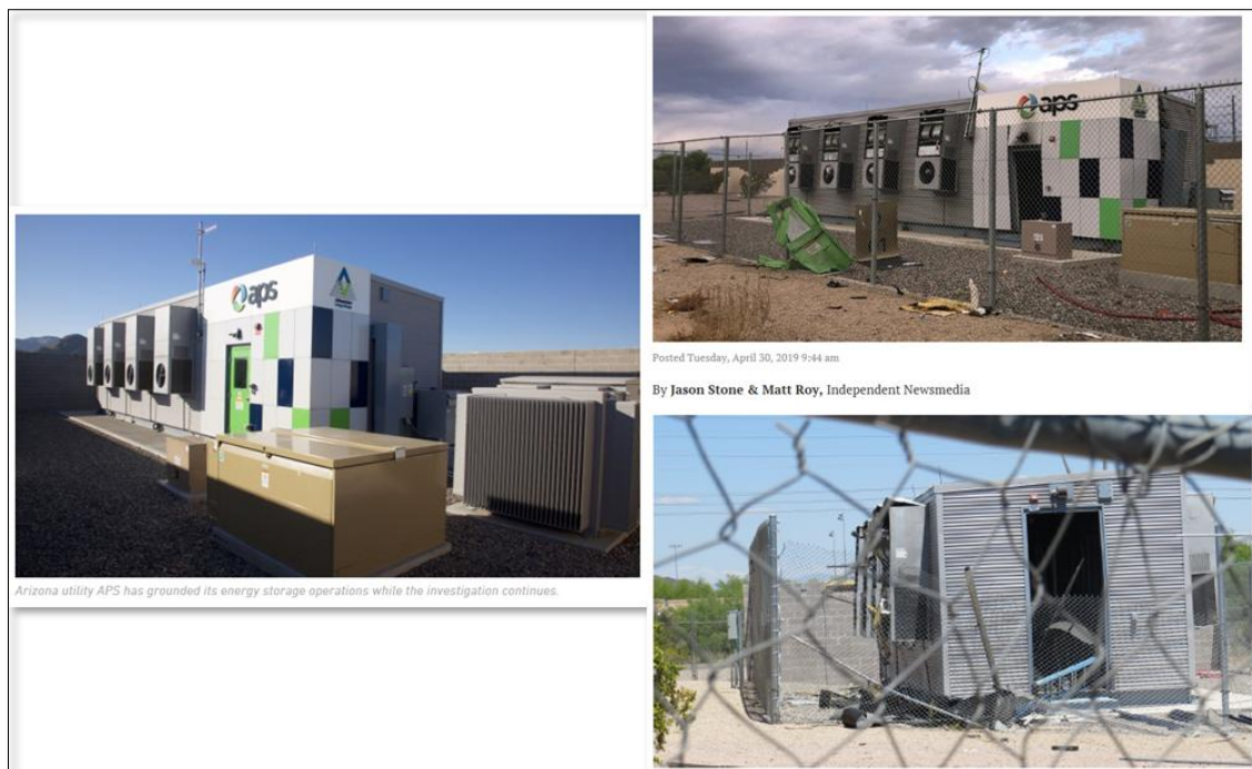
Figure 3.4.1 – Photo of lithium battery explosion scene
