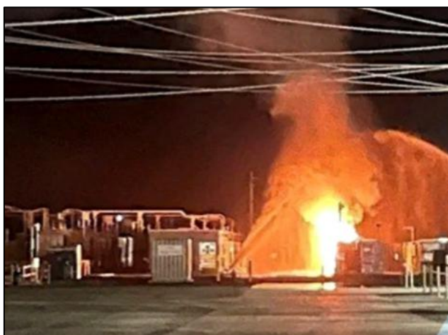
Figure 3.4.3 – Photo of Tesla Megapack fire scene
