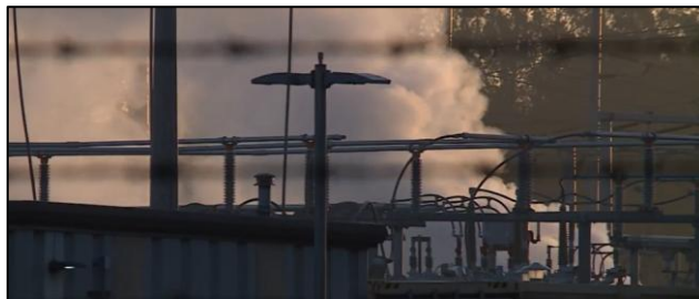
Source - Electric Power Research Institute
