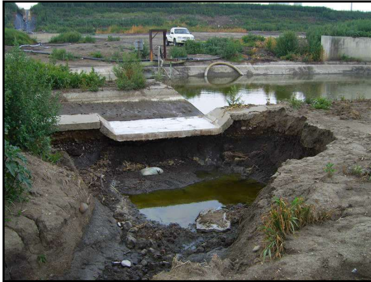
Figure 37 Erosion downstream of Fertiliser dam 8 due to overtopping
